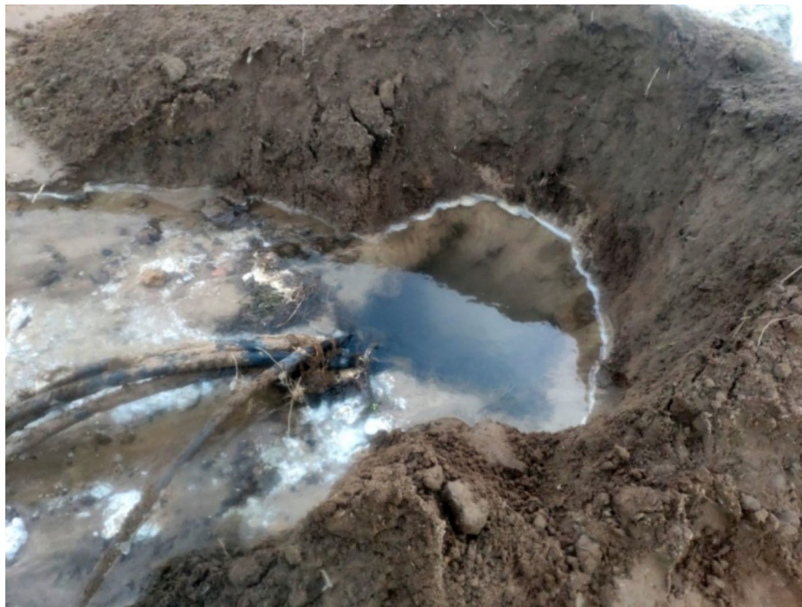
Fig. 13 Overflow of ~ 3 l/s in the village of Černěves
