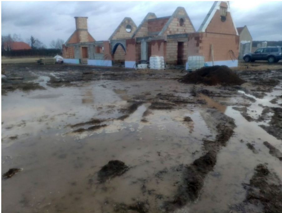
Fig. 14 Consequences of groundwater overflow
