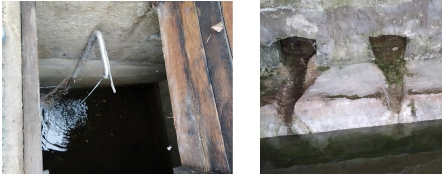
Fig. 20 Spring overflow in the village and water in the second spring on 24 October 2019
