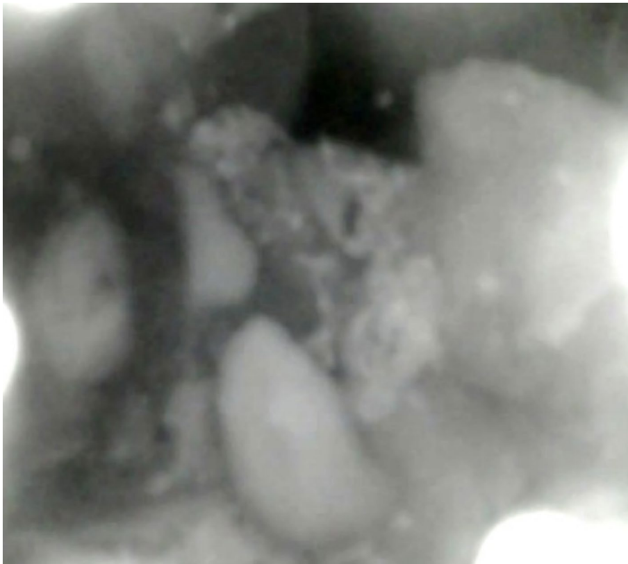
Fig. 21 Area of the hole (up) in the pipe of the ground heat exchanger (inner diameter 25 mm) at a depth of 40 m
