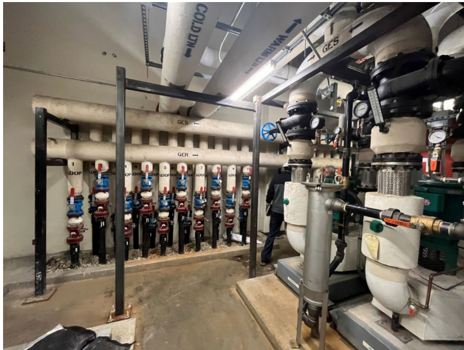
Fig. 9 Borehole array manifold in the plant room at the Calgary International Airport, May 2023. The manifold connects pipes to the borehole field for GHX arrays
