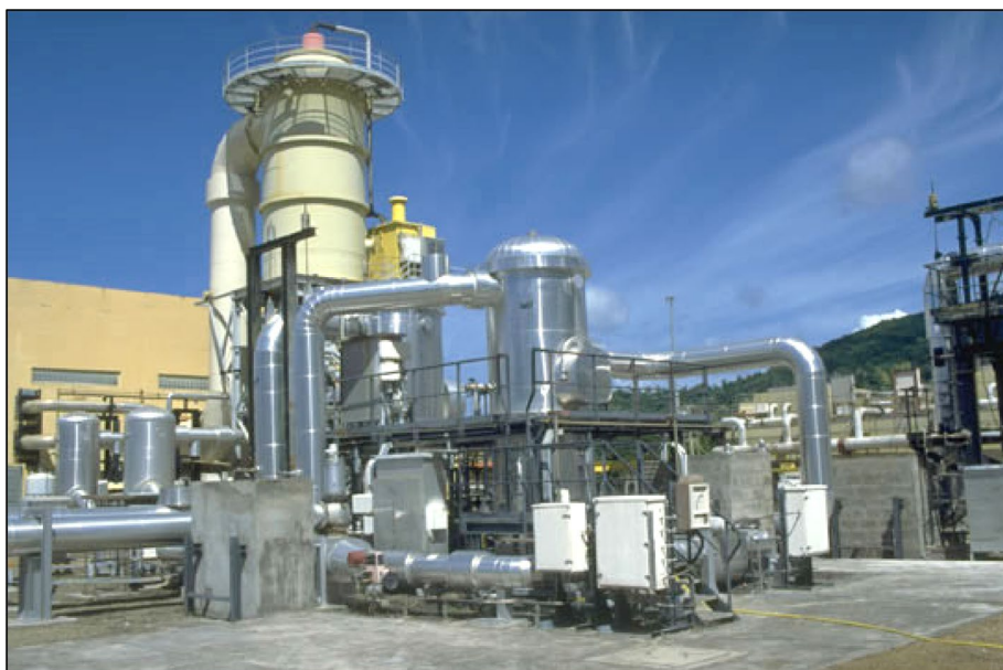
Fig. 6 View of the Bouillante 2 geothermal power plant at Guadeloupe Island (Credit: 2023 © Guadeloupe Energie. Taken from: https://www.guadeloupe-energie.gp/en/renewable-energy/geothermal-energy/the-geothermal-energy-sector-in-guadeloupe/ )
