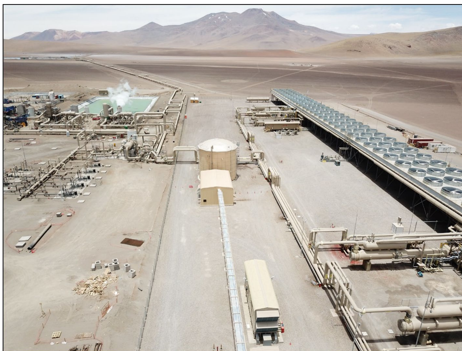
Fig. 5 View of the first power plant of Cerro Pabellón, Chile (Credit: ThinkGeoEnergy, 2018; https://creativecommons.org/licenses/by-nc/2.0/deed.en# )
